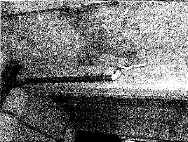
Dok L - Konkos imfaqqa (spalling concrete), kawzat minn ilma/drenagg minn bittha fis-sular ta' fuq (hsara giet imsewwija).
