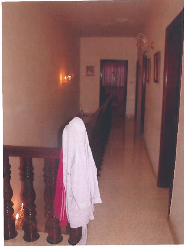
Paint on the underside of the ceiling of the corridor at the top floor is peeling off.
