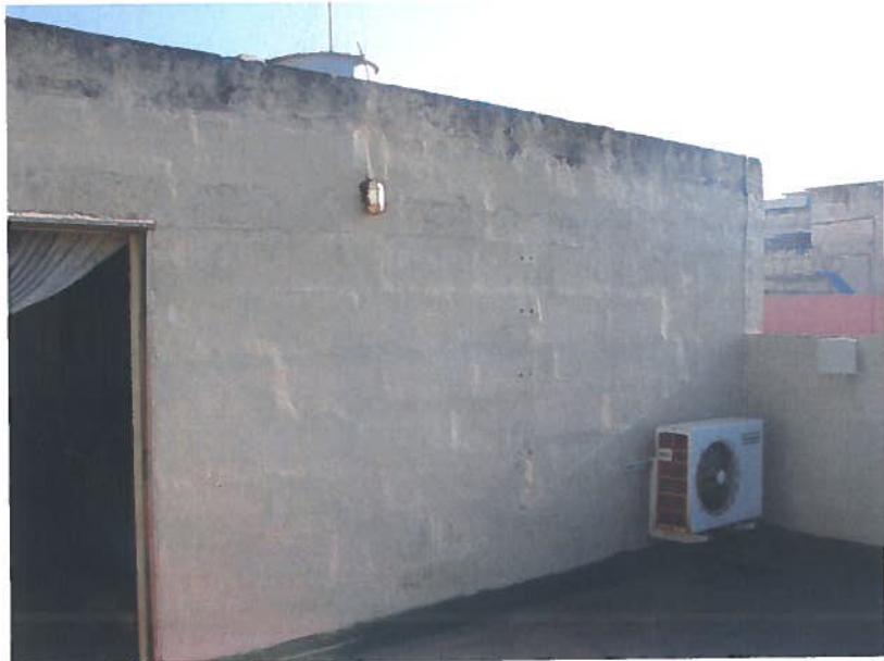
Washroom needs external plastering and painting.
