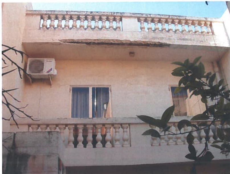
Areas of the overhang over the back terrace are spalling.
