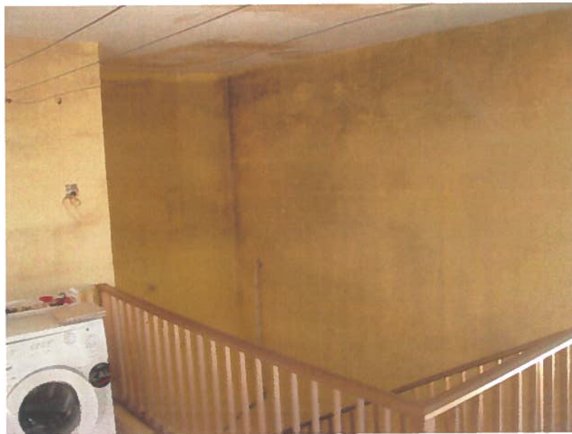
Signs of dampness are evident on the ceilings and walls of the washroom.
