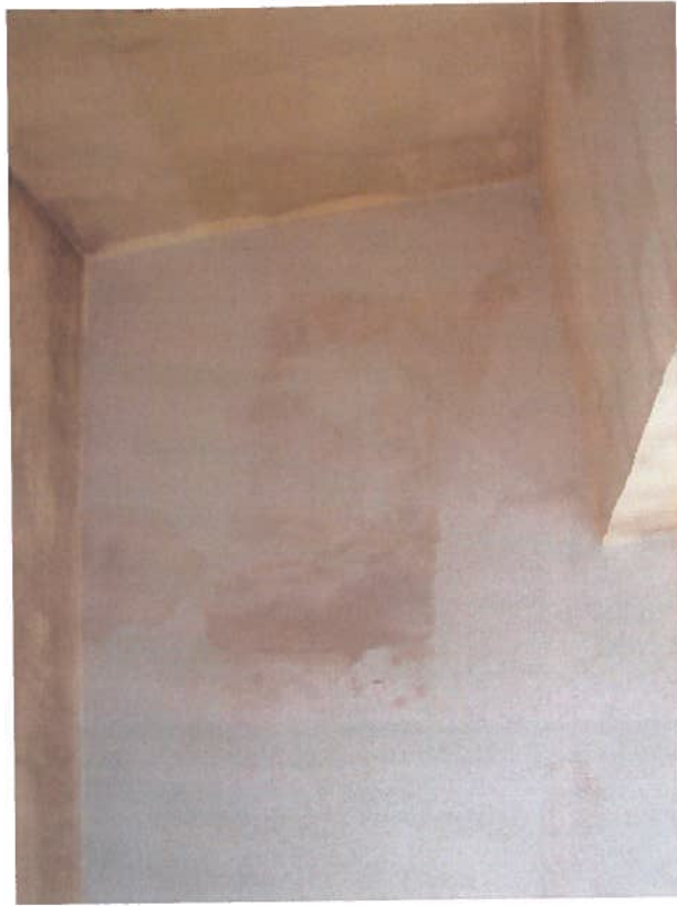
Further signs of dampness on the internal walls.
